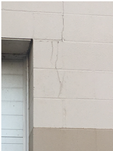
Figure 2: Differential movement in steel lintel within masonry wall
